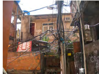
Electricity theft is illegal and also very dangerous due to the insecure connections and fire risks.
