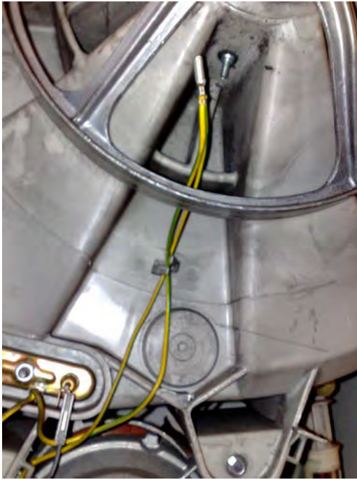
The green and yellow earth wire connected to the metal casing inside an electric motor.
