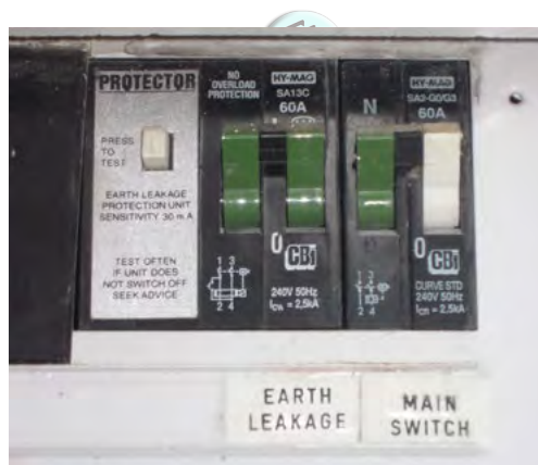
An example of the earth leakage and main switch on a distribution board in a house.
