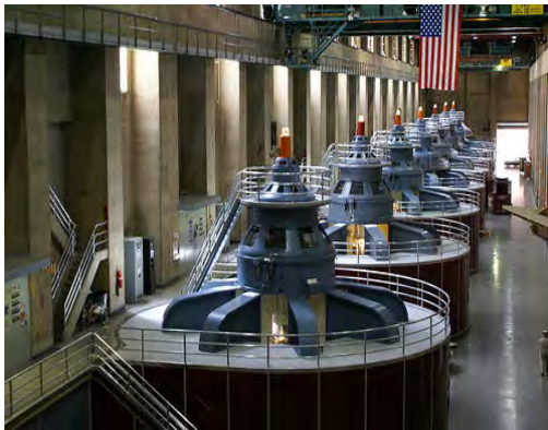
The generators inside the hydroelectric power plant.
