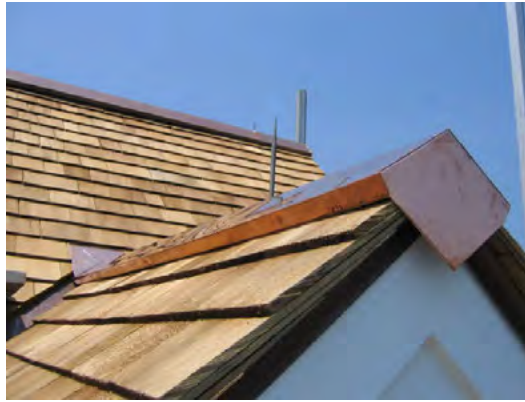
A lightning rod on the roof of a house.
