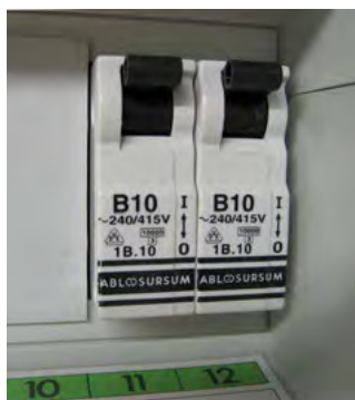
An example of circuit breakers showing the switches.
