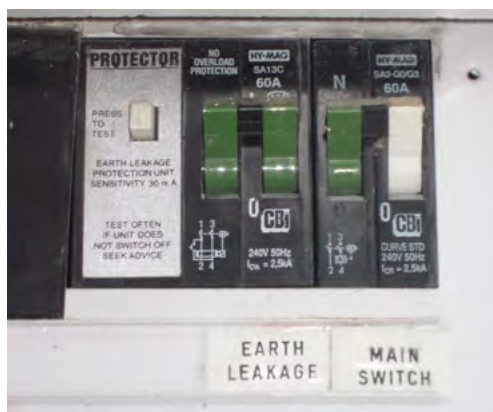
An example of the earth leakage and main switch on a distribution board in a house.
