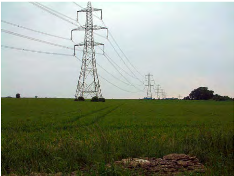
The national power lines transmit electricity across the country from the power stations.
