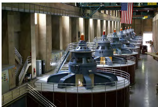
The generators inside the hydroelectric power plant.
