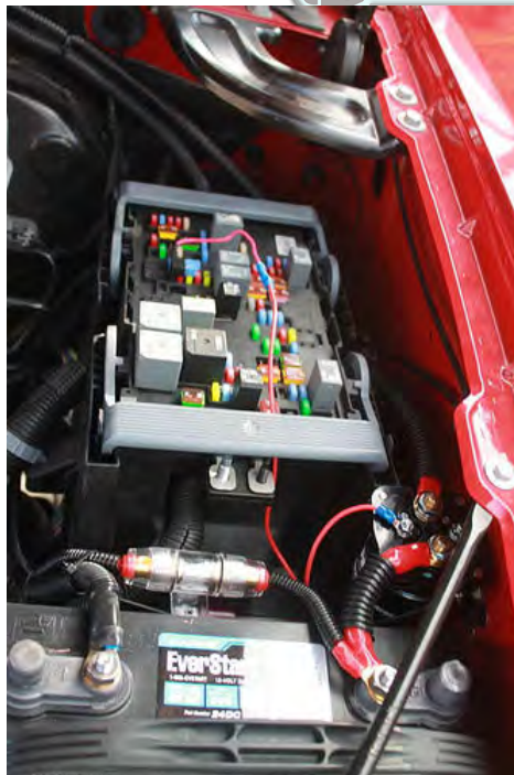
Motor cars also have fuses. Can you see the fuse in this photo showing the battery in a motor car?
